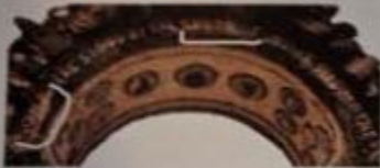
1. Letters on north arch face; left and right areas show deteriorated mortar.
