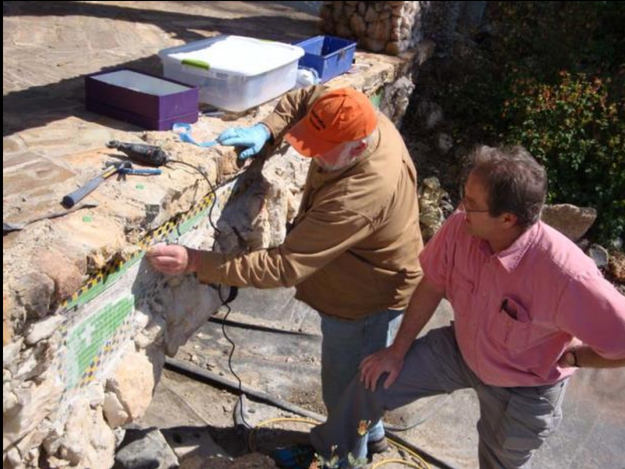
Conservator Don Howlett and trained Assistant David Van Allen inspect damage to mosaics on lower arch of bridge
