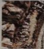
2. Area of dead mortar
