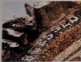
3. Deteriorated mortar joint above "BLESSED"
