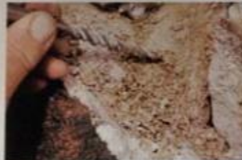
4. Extensive dead mortar on southwest arch face.
