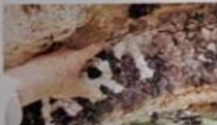
5. Deteriorating mortar at cold joint.
