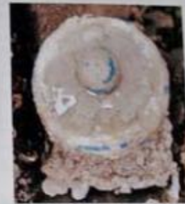
5. Failed Rockite used to attach tiles.
