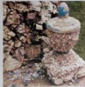
7. Detached tile and mirror, condition evident on all four ums.
